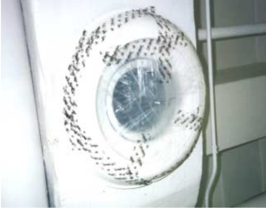
Figure 3. Sealed diffuser in Building LS-2
