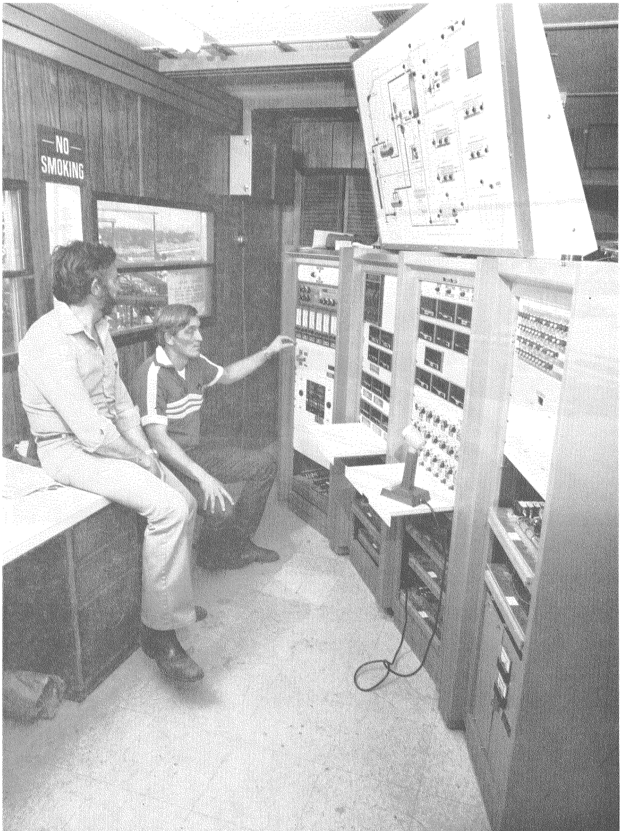
Fig. 30. 500 kW pilot plant control console.
