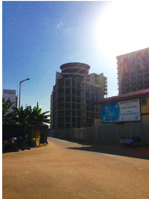
Figure 4: Airport City streetscape showing unfinished revolving restaurant, advertisement for Atlantic Tower, and informal kiosks
