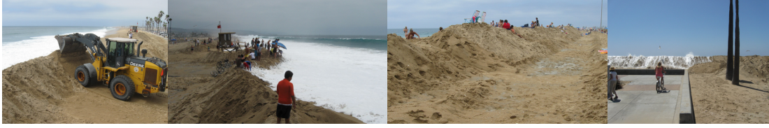
Figure 3.1: Anthropogenic berm such as these are constructed in the days and hours before an anticipated flood event in Southern California, and have been termed event-type berms by [Gallien et al., 2014].
