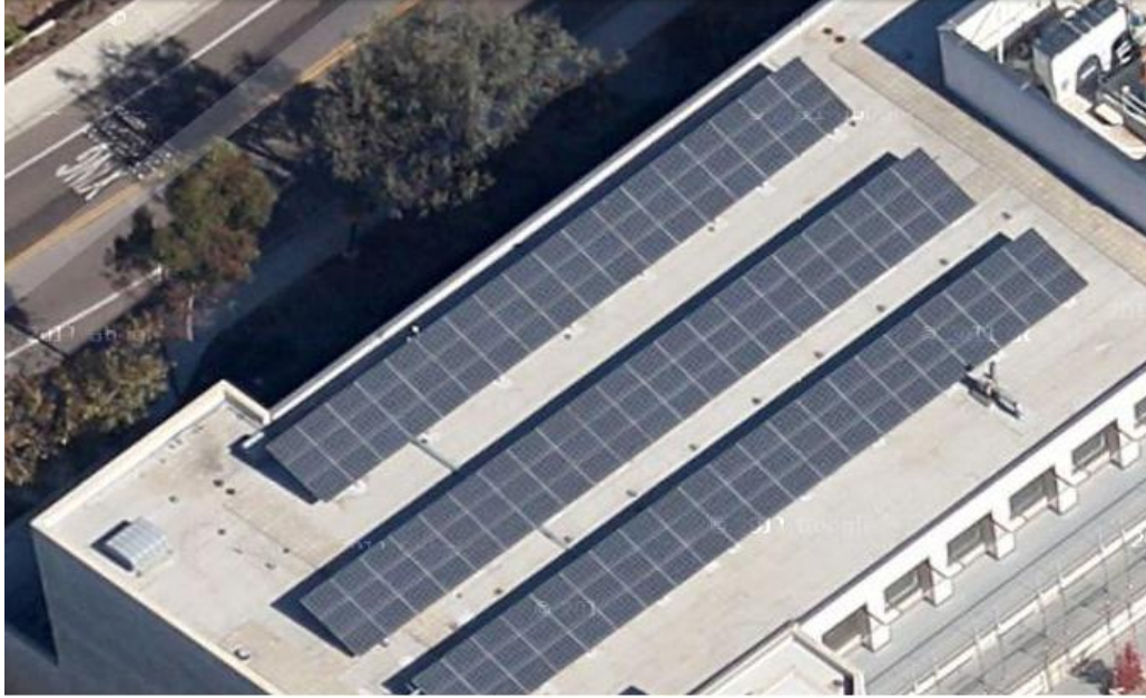
Figure 2: Aerial view of PV array and inverter system on the north side of Engineering Building Unit 2 (EBU2) located at 32.881324° North 117.232952° West (WGS84) (Map © 2011 Google – Map Data © 2011 Google)
