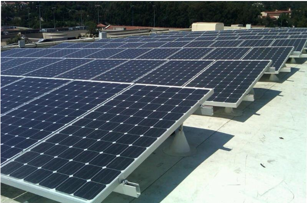
Figure 22 Solar panels on Ackerman Union's roof
