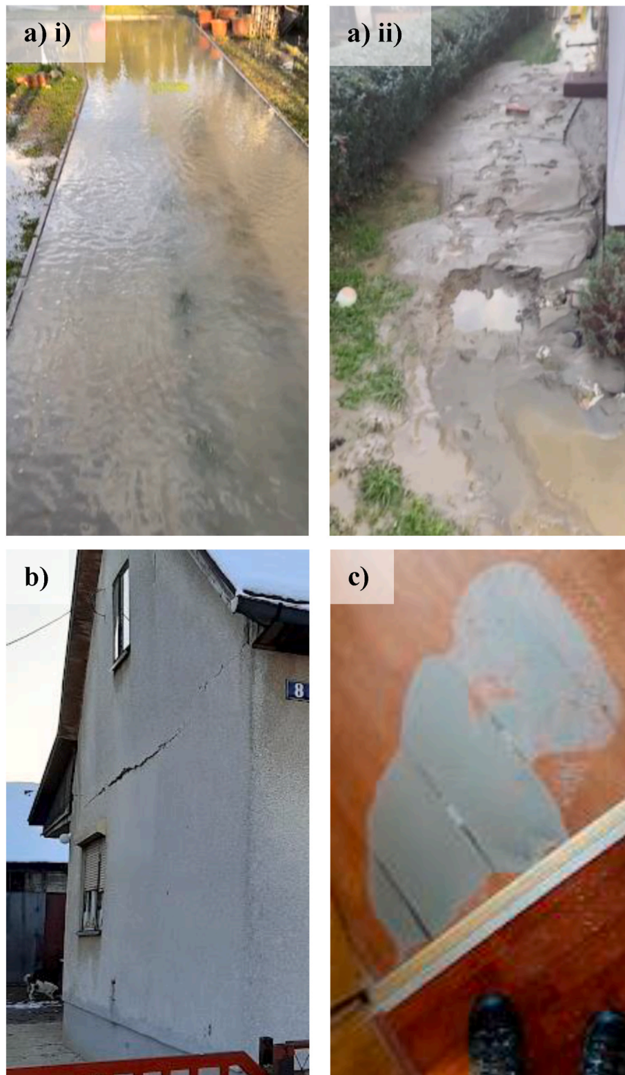
Fig. 6. Liquefaction effects at Milan Makanac St: (a) (i) liquefaction-induced flooding and (ii) sediment ejecta at 11 Milan Makanac St [45.4361N, 16.2629E], (b) structural damage, as evidenced by horizontal crack between the first story and the attic, at 8 Milan Makanac St [45.4359N, 16.2627E], and (c) ejecta inside the house at 10 Milan Makanac St [45.4358N, 16.2628E].
