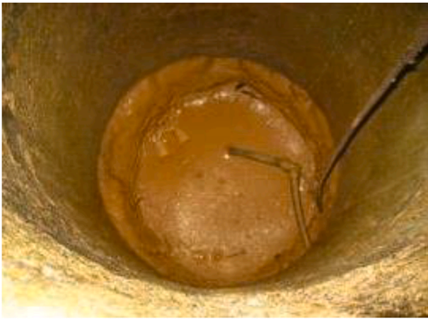
Fig. 7. Residential water well partially filled with liquefaction ejecta at Dre-nacka St, Petrinja [45.456224N, 16.316443E].
