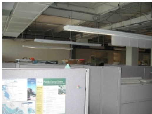
Figure 21. IBECS-Controlled Electric Lighting Fixtures.
