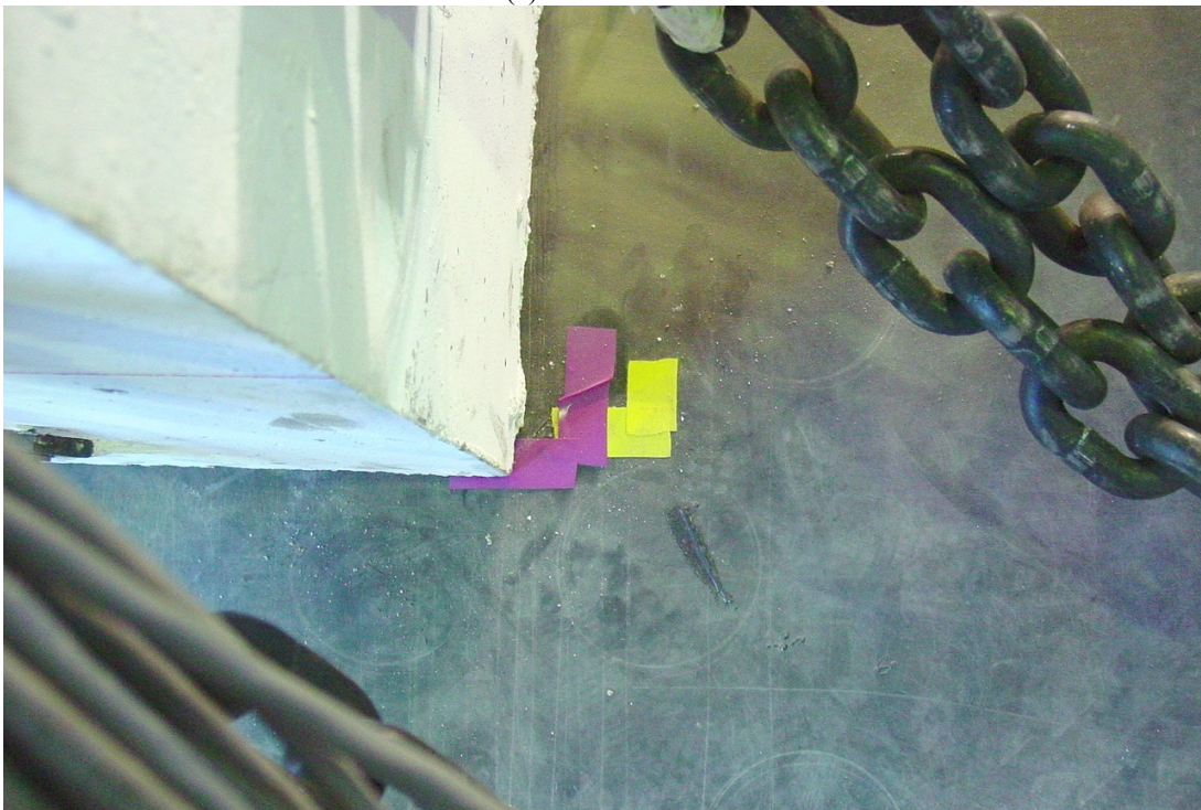
(b) Rotation about vertical axis indicated by distance from tape attached to elastomeric pad
