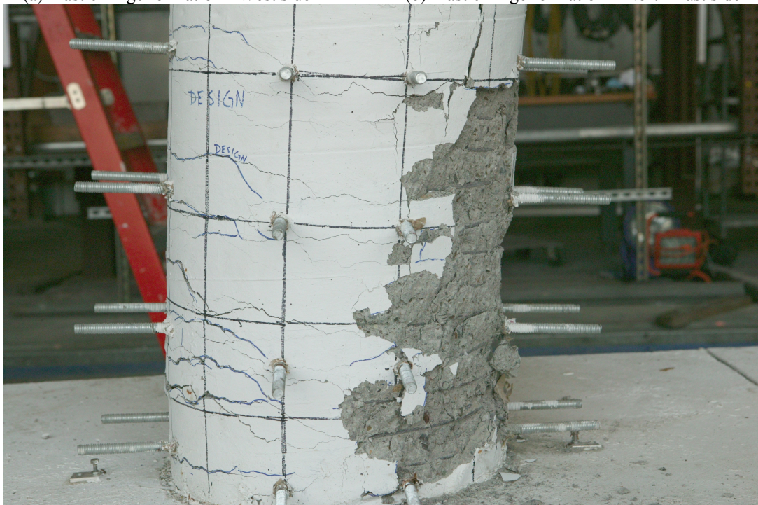
(c) Plastic Hinge formation – North side (after removal of instrumentation)
