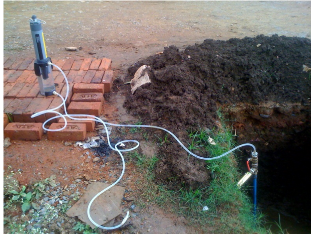
Figure 4.2: Sensors attached to direct tapping on pipe (Site: RADJ). YSI Sonde is on the left and Telog Line pressure monitor on the right.
