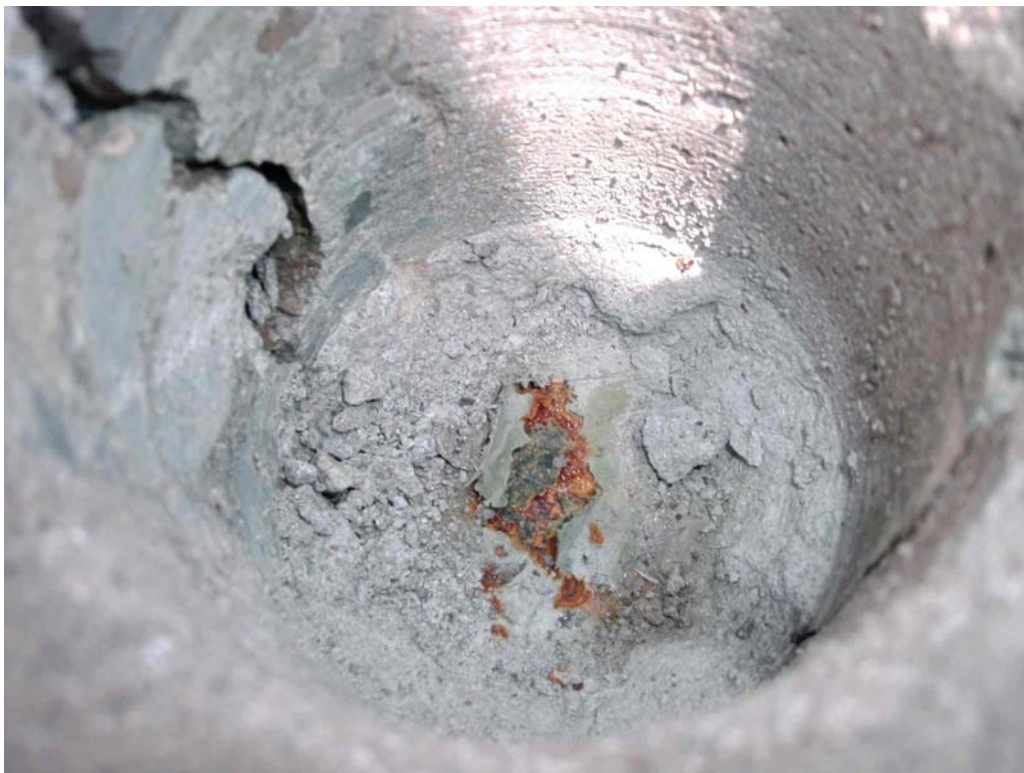
Figure 55. View of the interior of a recently made core hole showing corrosion products underneath the epoxy coating.
