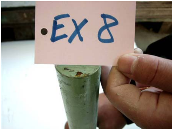
Figure 23. Corrosion on the epoxy-coated bars.
