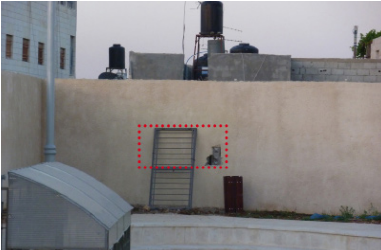
Image of the wall from inside the park (eastern border), the red dotted rectangle shows the former location of the window that I saw in my last visit in May 2011. (Iron frame was supposed to be placed on the window for protection).
