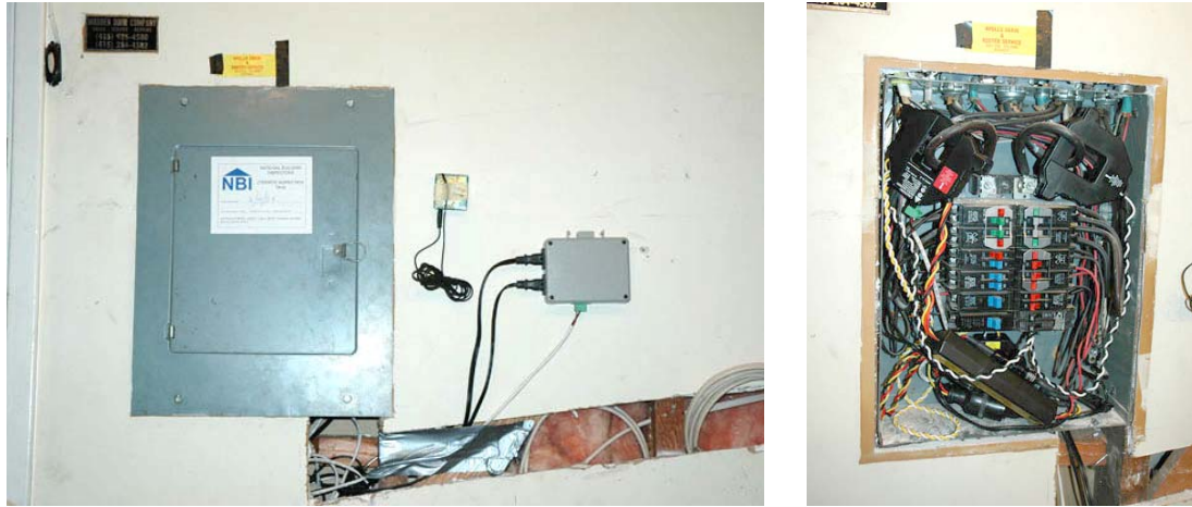
Figure 8: Left: Closed breaker box and mote enclosure. Right: Open breaker box showing CTs and communication cable.
