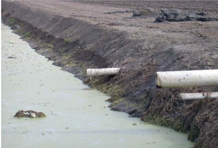
Perforated pipes or “tiles” drain water from the root zone of crops into adjacent ditches and other waterways.
