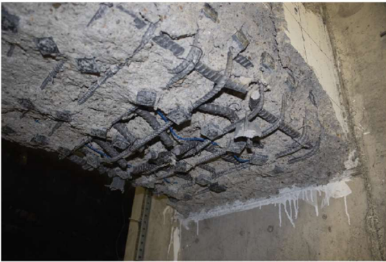
(g) Post-testing column-foundation joint (bottom face).
