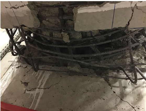
(i) Post-testing column-foundation joint (bottom face).
