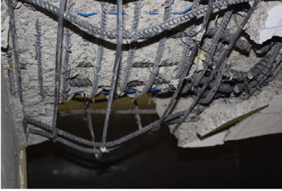
(g) Post-testing column-foundation joint (bottom face).
