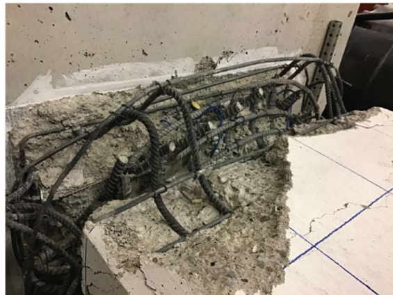
(j) Post-testing column-foundation joint (top face).
