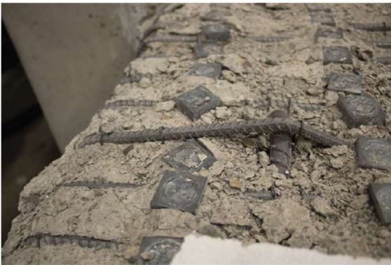
(q) Buckled transverse reinforcement. Note that the headed bar is not providing an effective restraint on the hoop.
