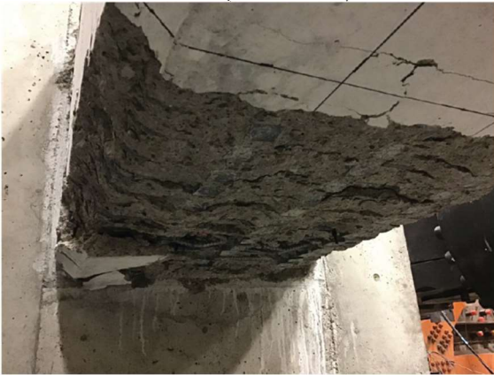
(o) Post-testing column-foundation joint (bottom face).
