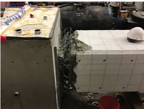
(e) Post-testing column-foundation joint (south side).
