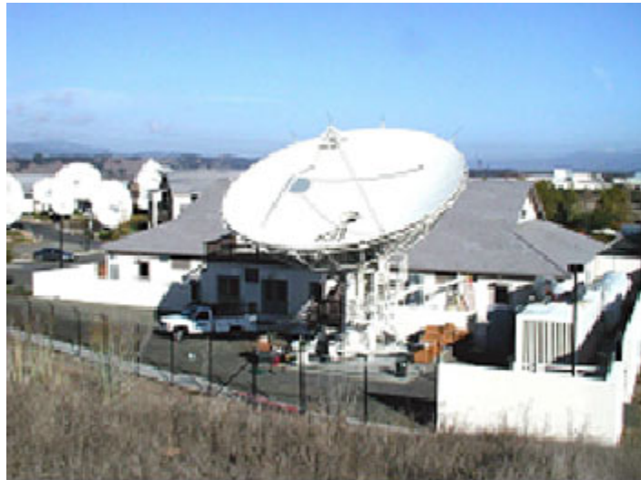
Figure 4.39 Recently installed WAAS Ground Uplink Facility in Napa California [SatNav,2005].
