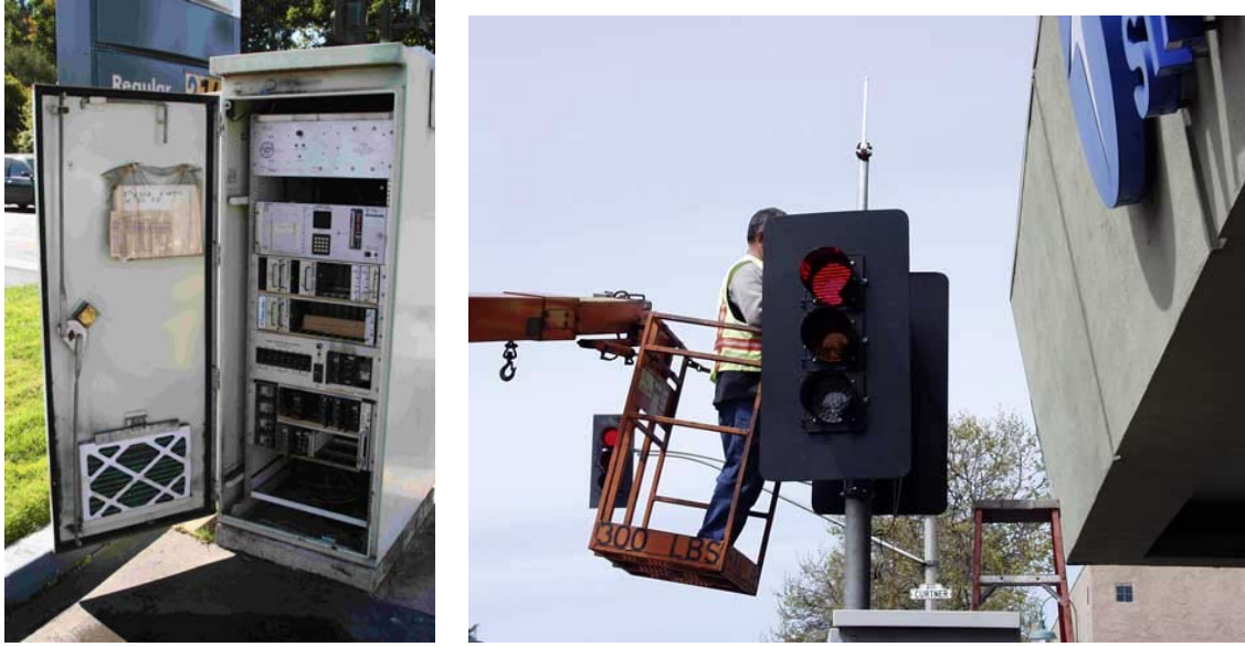
Figure 4.51 RSE cabinet and wireless communications antenna installation [VII CALIFORNIA, 2006b, c].
