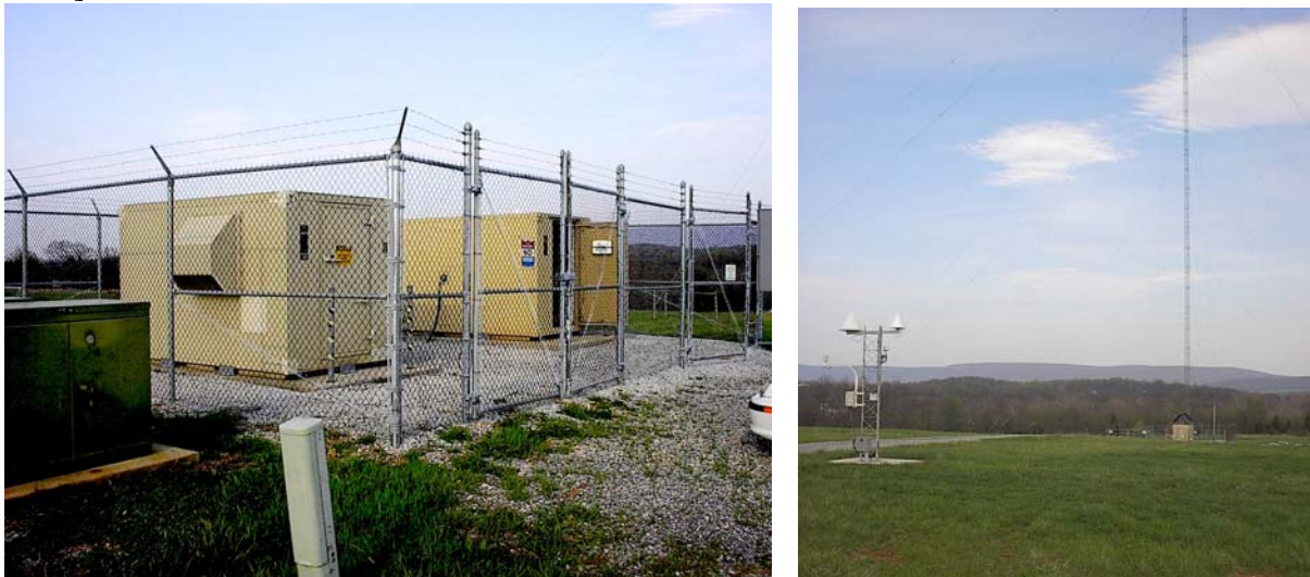
Figure 4.40 USCG NDGPS broadcast site [FHWA, 2005].
