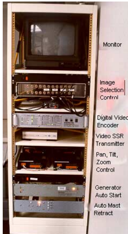
(b) Right equipment rack
