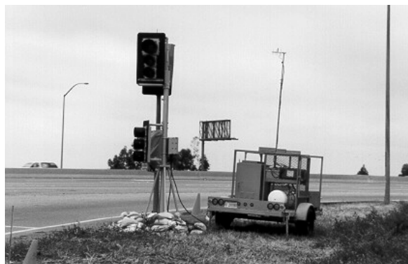
(c) Ramp meter trailer and signal
