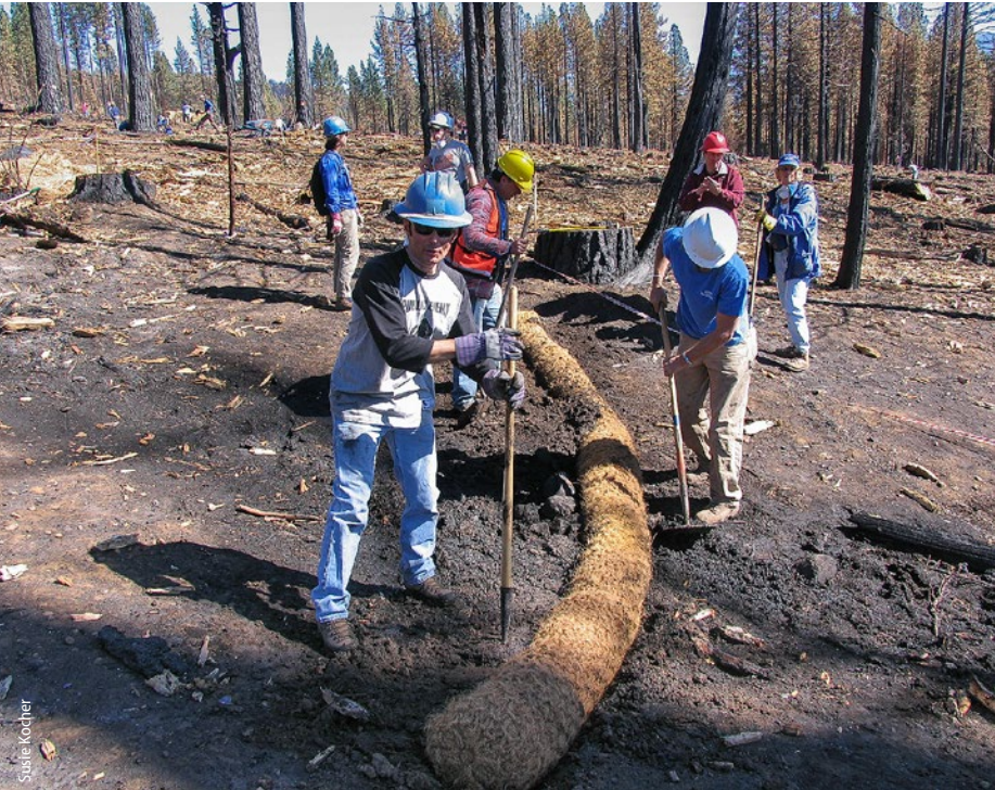
Volunteers for the League to Save Lake Tahoe install erosion control measures following the 2007 Angora fire near South Lake Tahoe. The fire burned 3,100 acres, destroying 250 residences.
