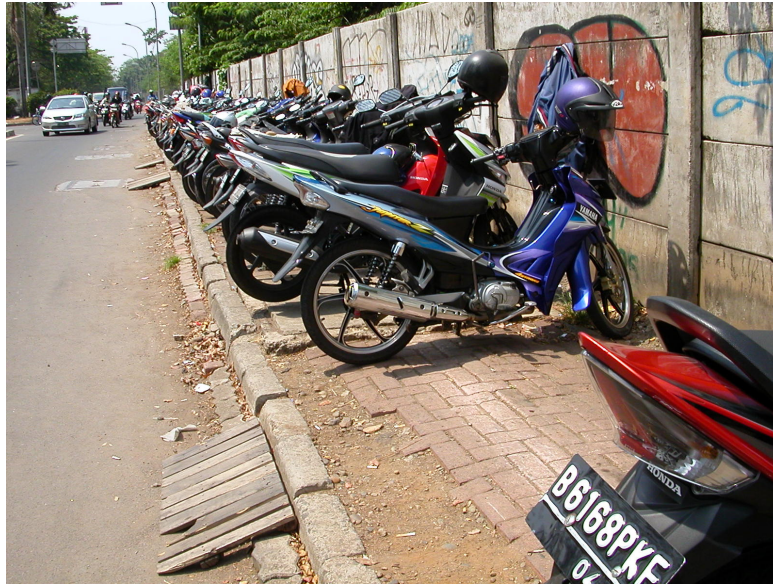
Figure 13: Sidewalk encroachment and damage by vehicle parking in Central Jakarta
