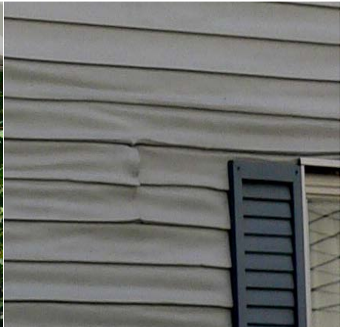
Figure 1b. Vinyl siding with more common, less severe, distortion
