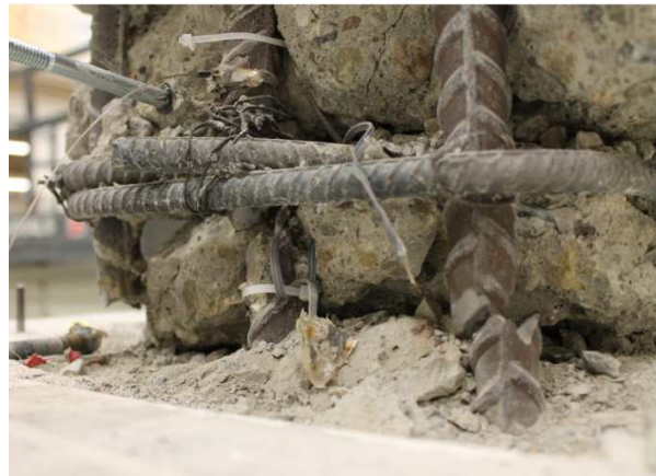
Figure 4.3.3: Failure Mechanism of SBL100 by Fracture of Longitudinal Bars
