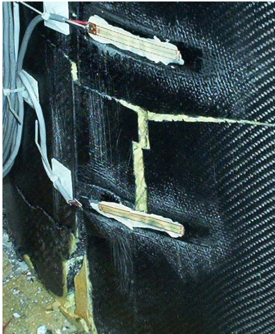
Figure 3-54: Jacket Splitting at Seam
