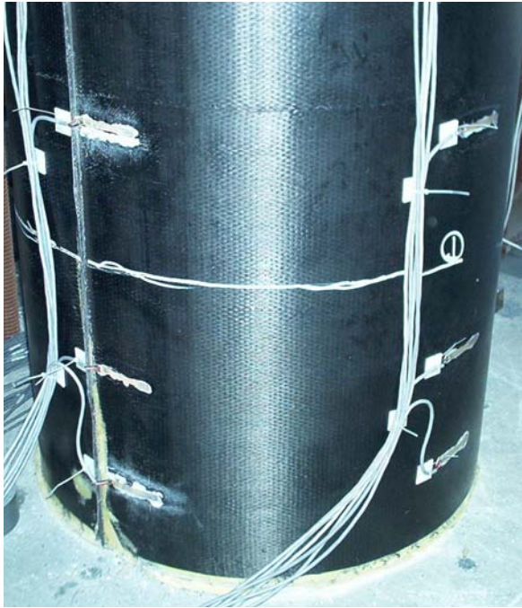
Figure 5-21: Composite Jacket Breaking in Hoop Direction of Column
