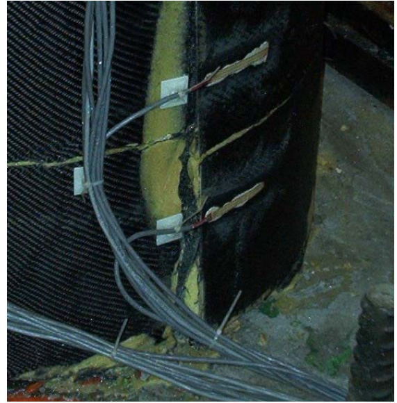
Figure 3-30: Jacket Splitting at Seam
