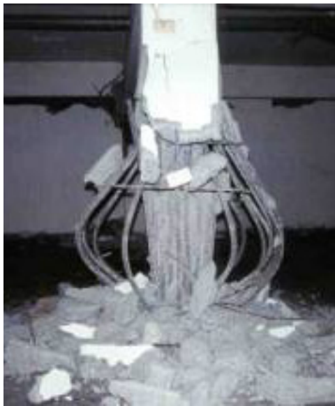
Figure 1-14: Non-ductile Column Failure [37]
