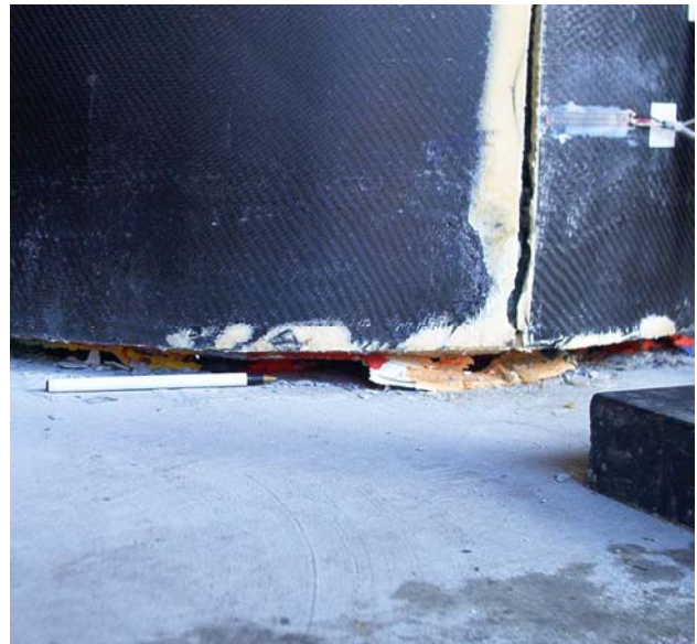
Figure 5-46: Jacketed Column Rising Up Creating Gap with Concrete Base
