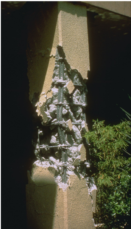
Figure 1-19: Column Shear Failure [37]
