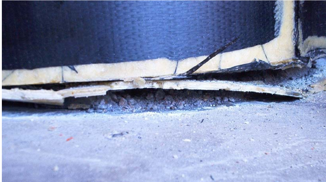
Figure 5-20: Lifting of the Column from the Footing during Testing
