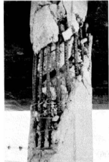
Figure 1-3: Foothill Freeway Column Failure [2]
