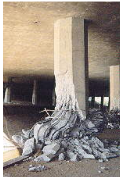
Figure 1-15: Non-Ductile Column Failure [37]
