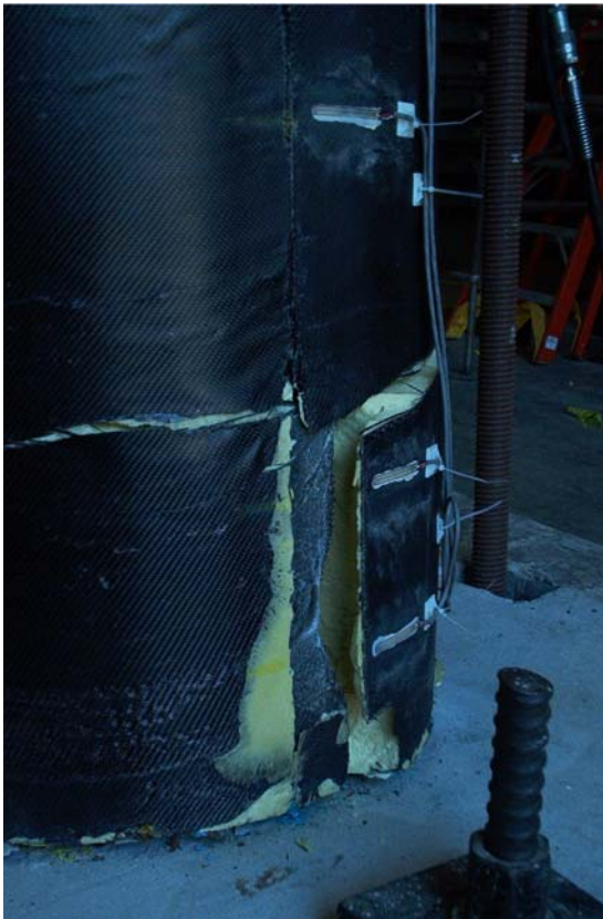
Figure 4-51: Square Column Jacket Failure
