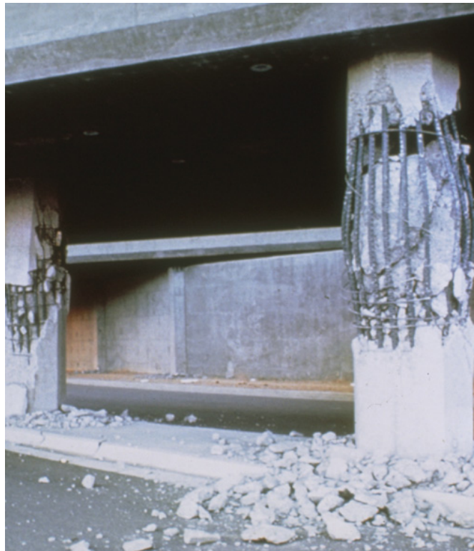
Figure 1-20: Column Shear Failure [37]
