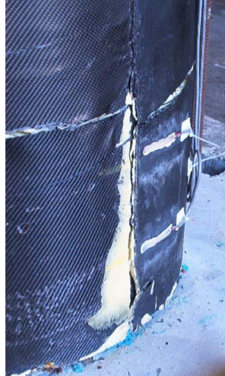
Figure 4-46: Jacket Splitting at Seam
