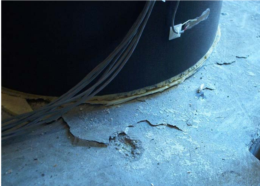
Figure 5-27: Concrete Base Cracking and Spalling
