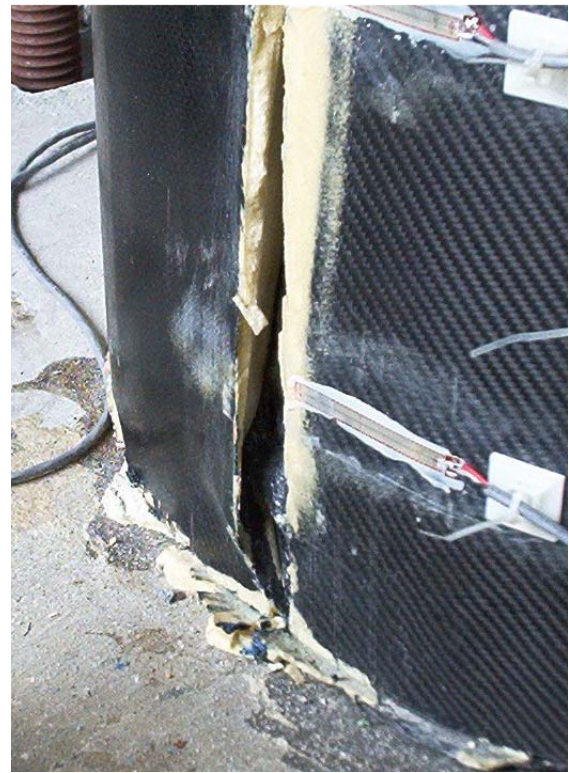
Figure 4-23: Jacket Splitting at Seam
