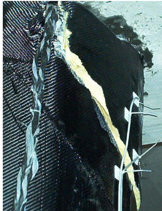
Figure 3-55: Jacket Splitting at Seam
