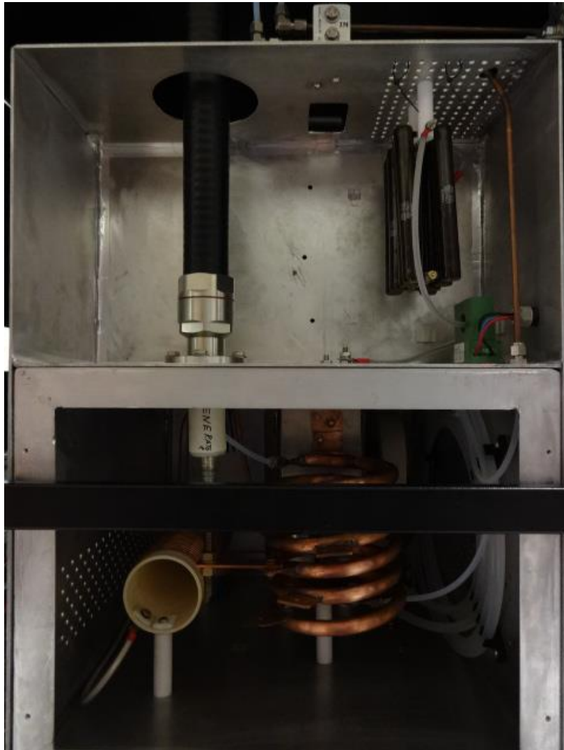
Fig. 10 – Inside the right panel of power supply. Cooling water lines are visible on right side near the copper coil. The cooling water flowing to and coming from the capacitor bank box are visible at the very top center of the image.
