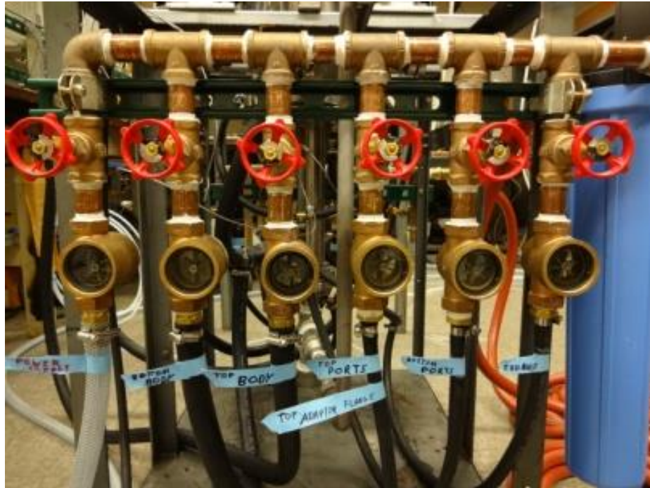
Fig. 3 – Source manifold for cooling water. Blue water filter is seen on the right.
