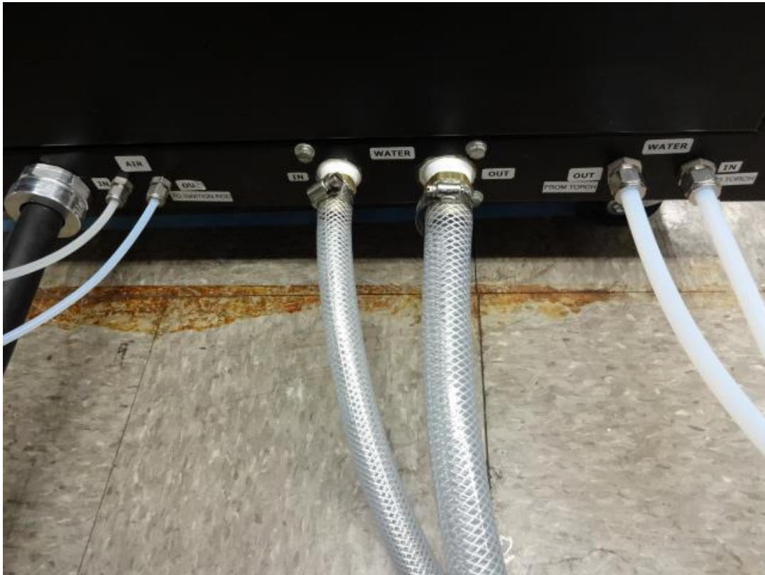
Fig. 4 – Bottom of back panel of power supply. (From left to right: 480 V 3-phase cord, compressed air in from gas cylinder, compressed air out to ignition rod, main cooling water inlet, main cooling water outlet, cooling water from torch, cooling water going to torch)
