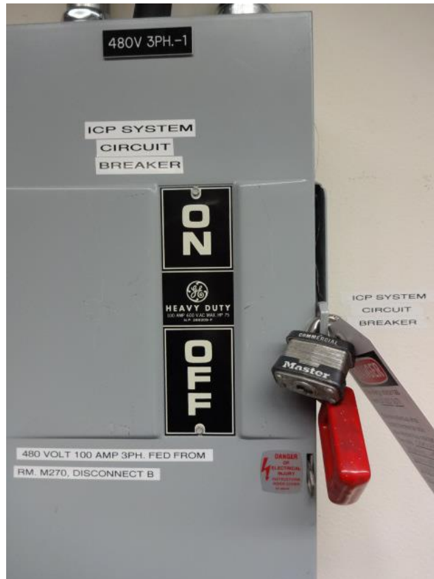
Fig. 11 – Main EPIC system circuit breaker. (Here the breaker is switched off and has been locked out.)
