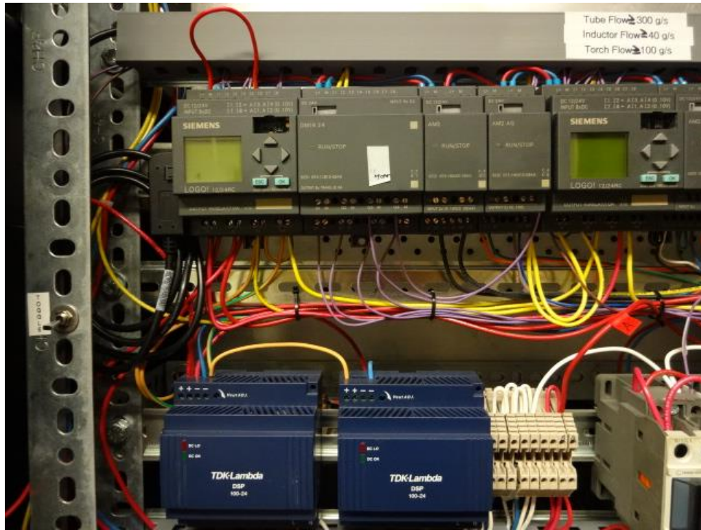
Fig. 13 – Inside the front panel of the power supply. The Siemens screen on the left is used to read U_a , I_a , I_{grid} , T_r (and is duplicated on the LOGO module screen on the front panel). The Siemens screen on the right displays cooling water temperatures and flows. To change between the two, use the switch on the left labeled “TOGGLE.”
