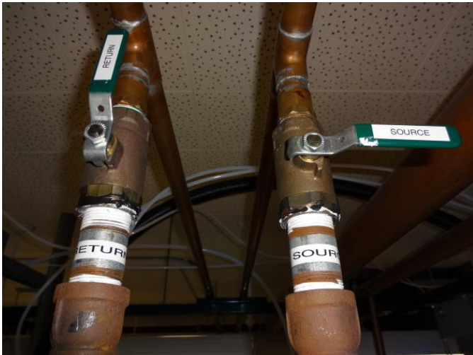
Fig. 1 – Source and return valves near ceiling pipe for cooling water. (Here return valve is open and source valve is closed.)
