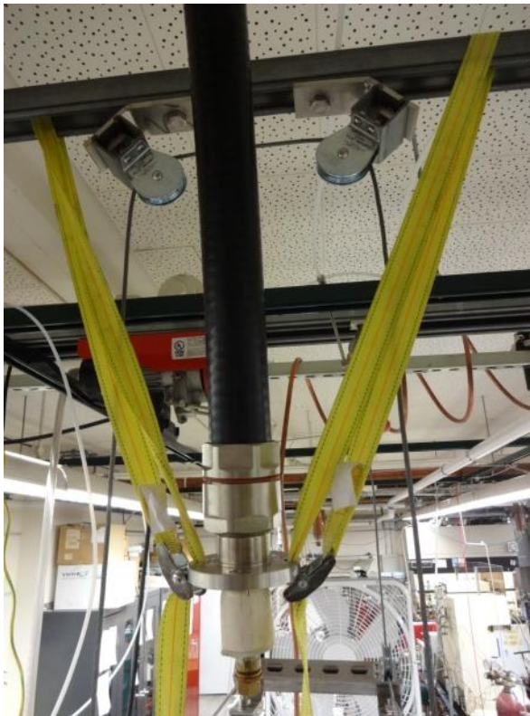
Fig. 20 – High voltage power line secured to unistrut ( image taken after torch has been lowered ).
