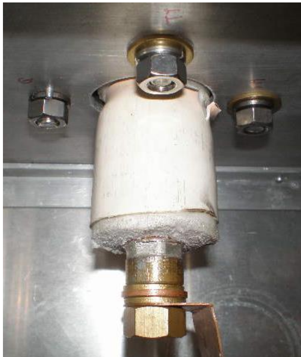
Fig. 19 – High Voltage Power Line connection to capacitor bank and torch. ( Located inside the capacitor bank box ).
