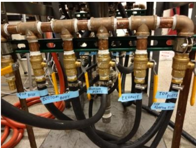
Fig. 2 – Return manifold for cooling water. (Here all labeled valves are open and valve furthest left is closed.)
