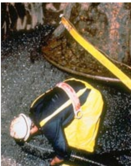
Worker removing zebra mussels from water intake pipes. Photo: Ron Peplowski, Detroit Edison—Monroe, Michigan Power Station
