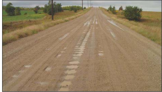
Figure 5.8: Insufficient crown (<4 percent).
