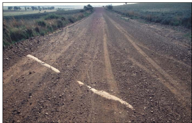
Figure 3.2: Poor gravel road (note cross-drain pipe exposed after excessive gravel loss).
