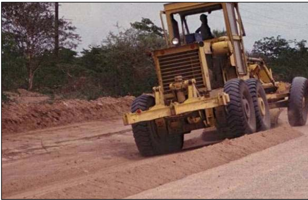
Figure 5.9: Too much crown (>6 percent).
