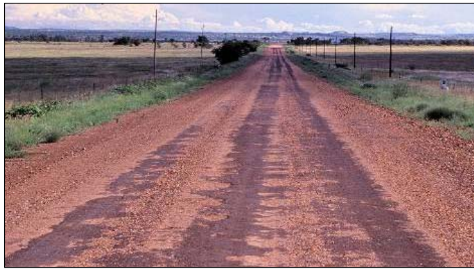
Figure 5.2: Insufficient chemical treatment application.
