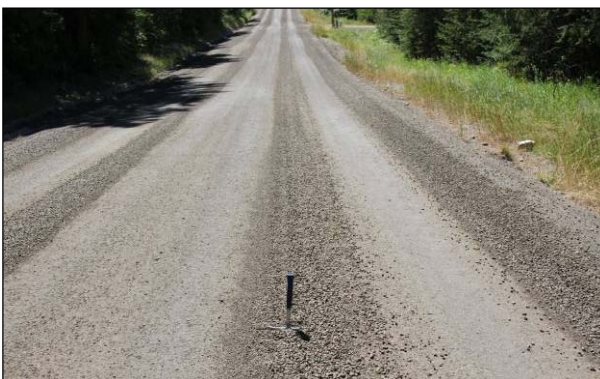
Figure B.13: Raveling.
