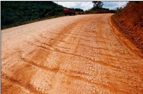
Figure B.8: Transverse erosion.
