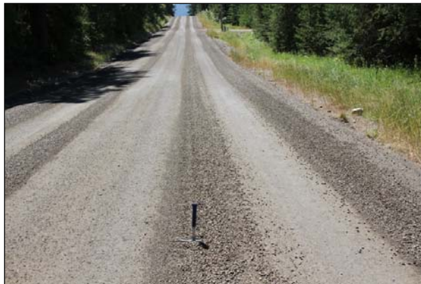
Figure B.21: Raveling on road surface after applying a chemical treatment.
