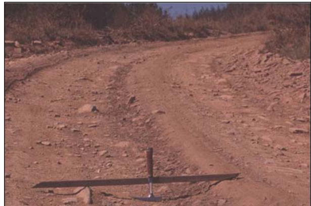
Figure 1.5: Unsuccessful attempt to fix a bad road with a chemical treatment.
