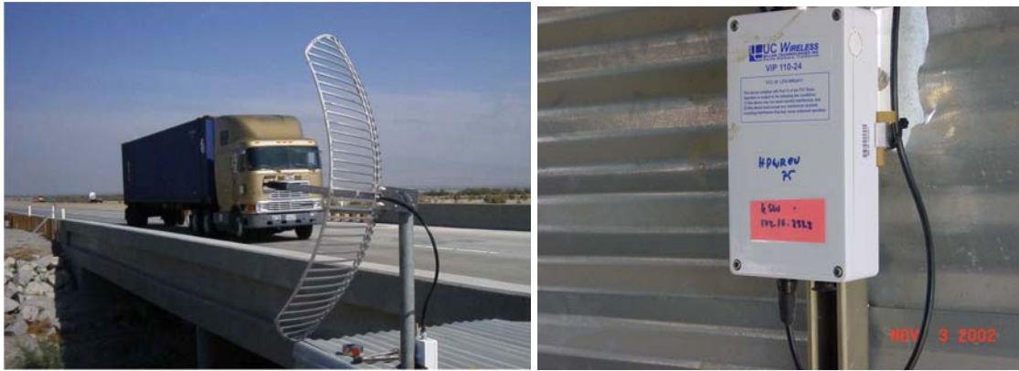
(a) Wireless Antenna
