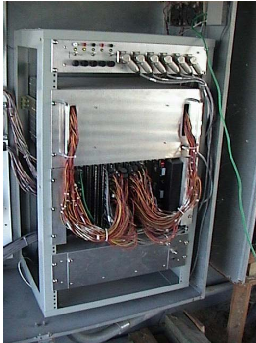
Figure 6-28 Data Acquisition Equipment Cabinet
