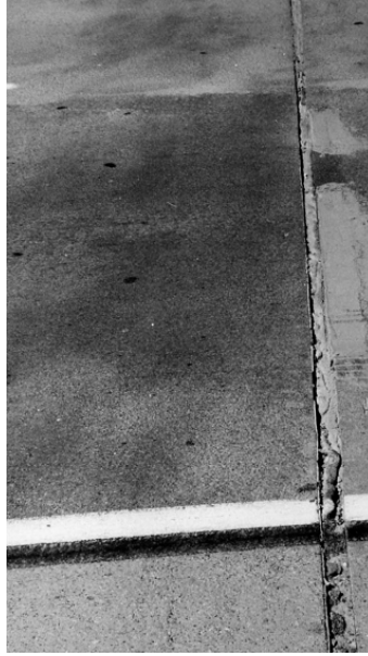
Figure 6-75 Weakened Expansion Joints
