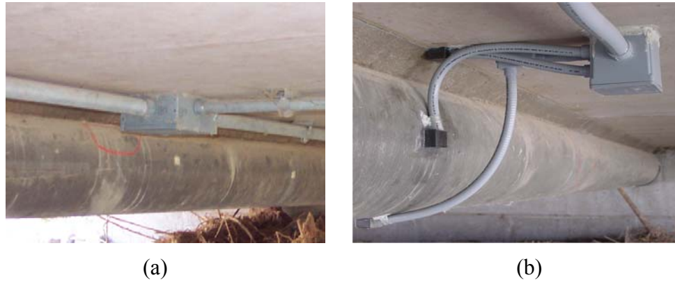
Figure 6-24 Instrumentation Housing and Conduit: (a) Accelerometer Housing (b) Strain Gage Housing and Conduits
