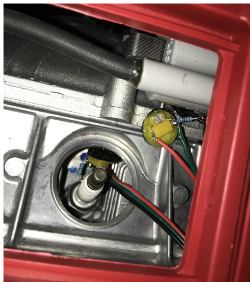
Figure 2.12: Photoresistors velcroed into the spark plug cover and spark plug cap of the generator.
