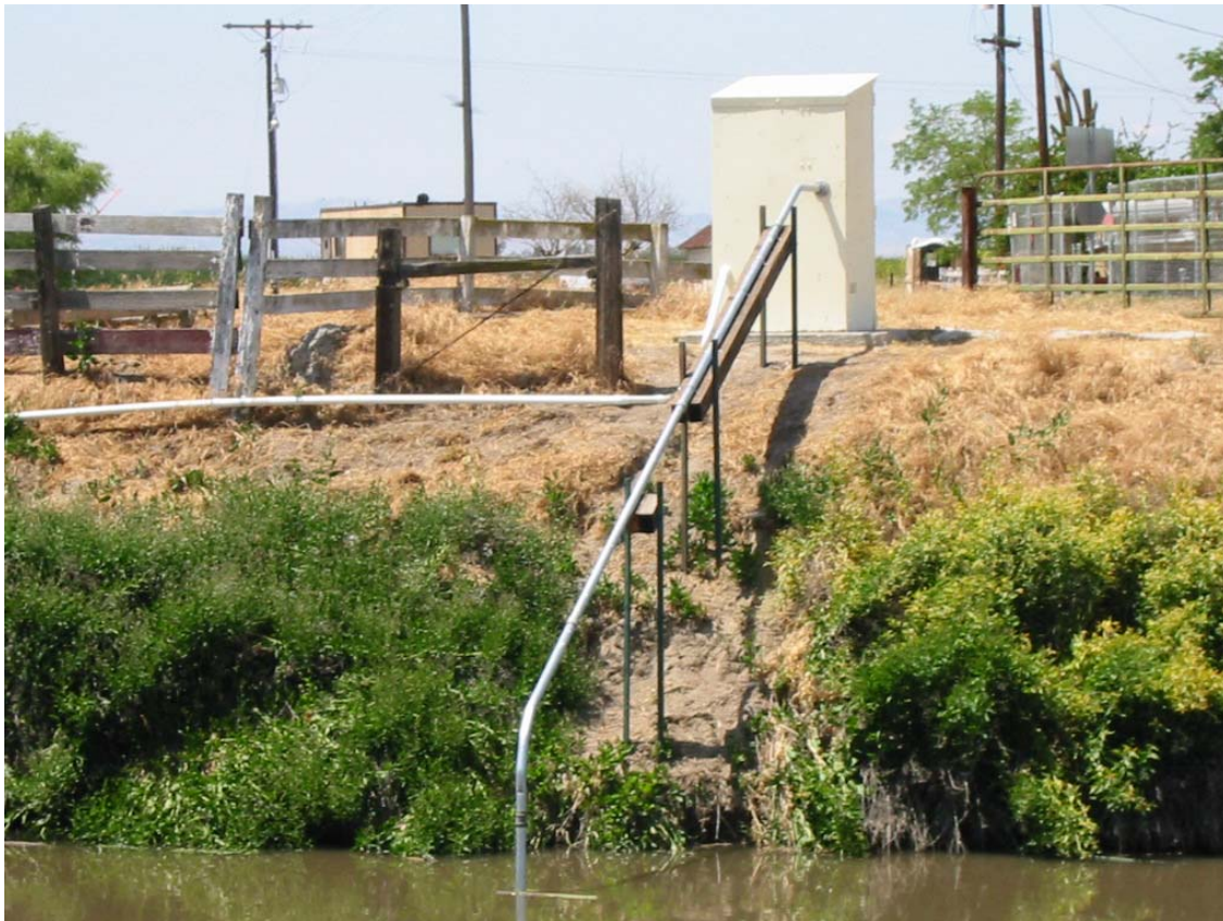
Figure 10. Example of a station installed at Wolfsen Road Bridge showing protective piping to house sensors and avoid damage due to vandalism. This site benefited from close access to power and a telephone line which avoided the cost of a solar panel and expensive telemetry.
