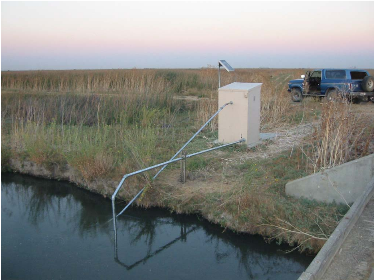
Figure 11. Installation in Volta State Wildlife Area showing the use of a solar panel mounted above the gauge house to power the sensors. This site suffered from frequent vandalism resulting in frequent damage to the velocity and electrical conductivity sensors. This was overcome using heavy gauge water pipe through which the sensor could be lowered into the water. The cable was secured inside the gauge house to prevent the sensor from being pulled further than a few inches beyond the submerged end of the sloping pipe.
