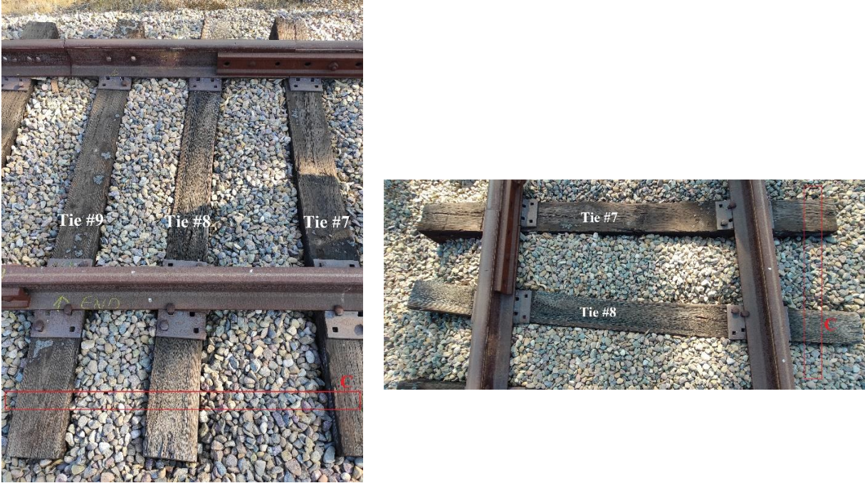
Figure 2.17: Misalignment of tie #8. The box denoted by ‘C’ shows the area scanned by the camera.
