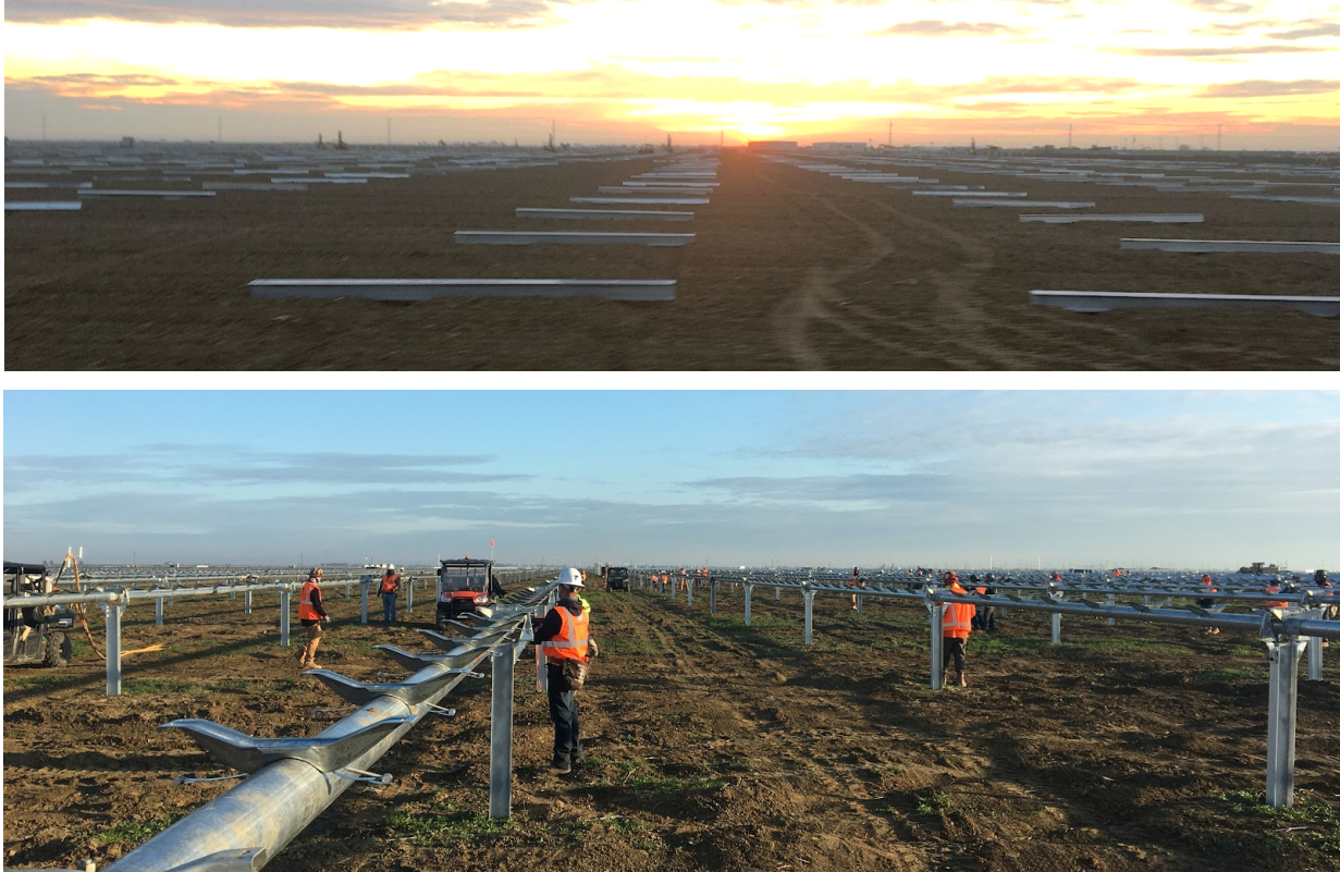
Figure 1. Building Aquamarine Solar. (Author, 2021)
