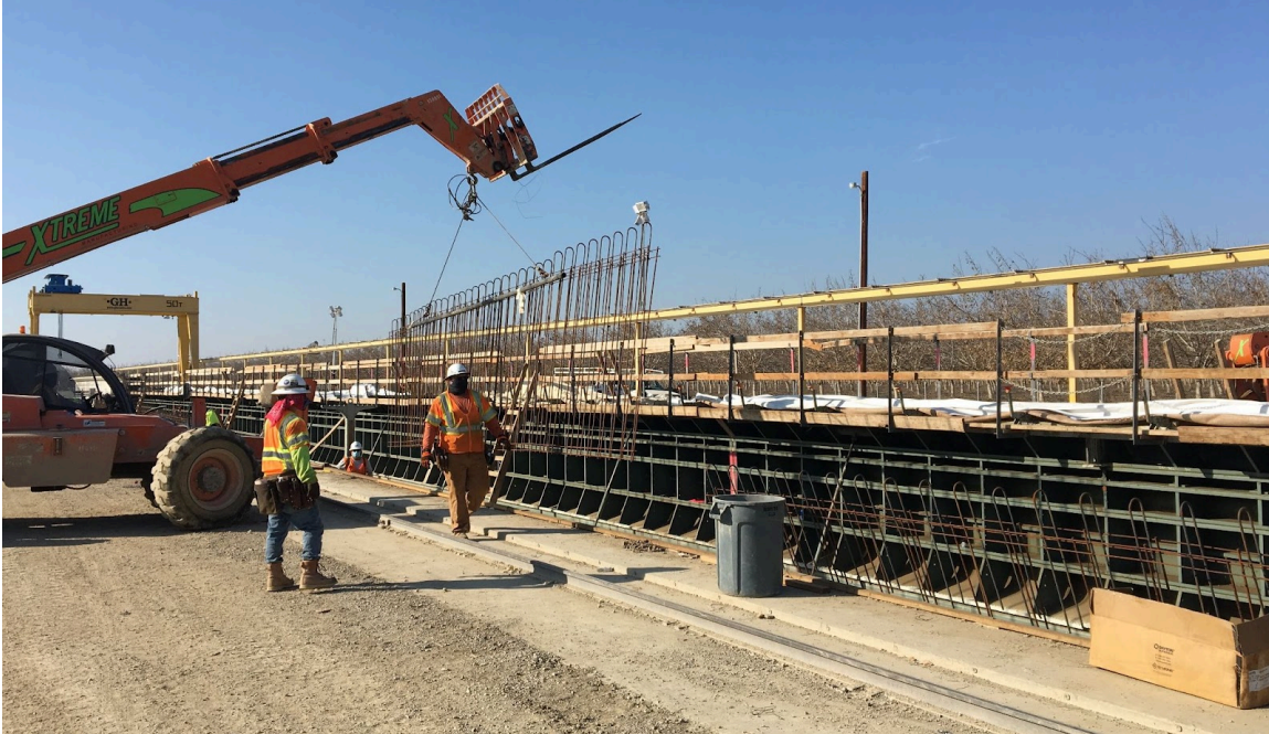
Figure 7: A pre-fabrication plant for high speed rail platforms and towers, near Hanford, CA. (Author, 2020)
