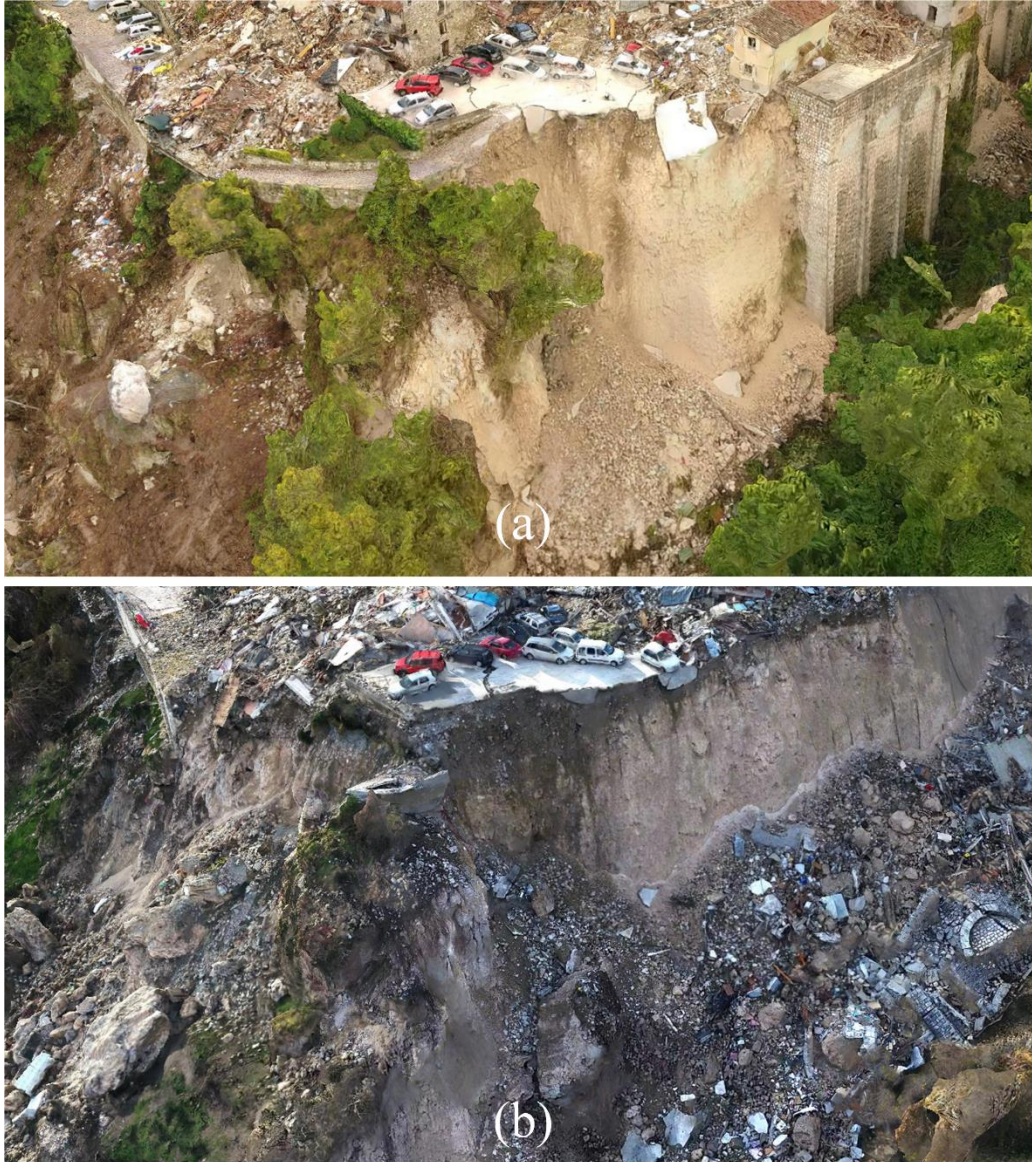
Figure 9. 3D mesh model images of the debris slide and retaining wall collapse below the village of Pescara del Tronto (a) following the August 24 th event, and (b) following the October 30 th event
