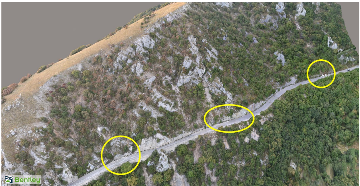
Figure 4.19. 3D model image of the SP 477 rockfall. Visible rocks and debris on the road are circled in yellow (42.7661 N 13.1669 E).
