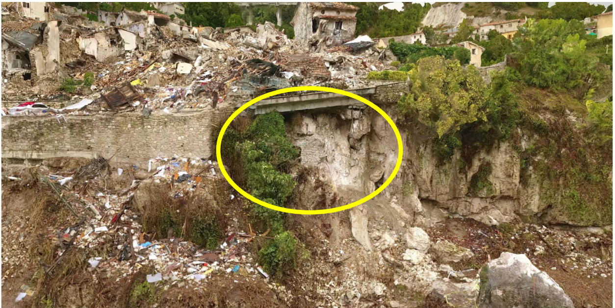
Figure 4.26. 3D model image of retaining wall damage from landslide below Pescara del Tronto (42.75057 N 13.27223 E).
