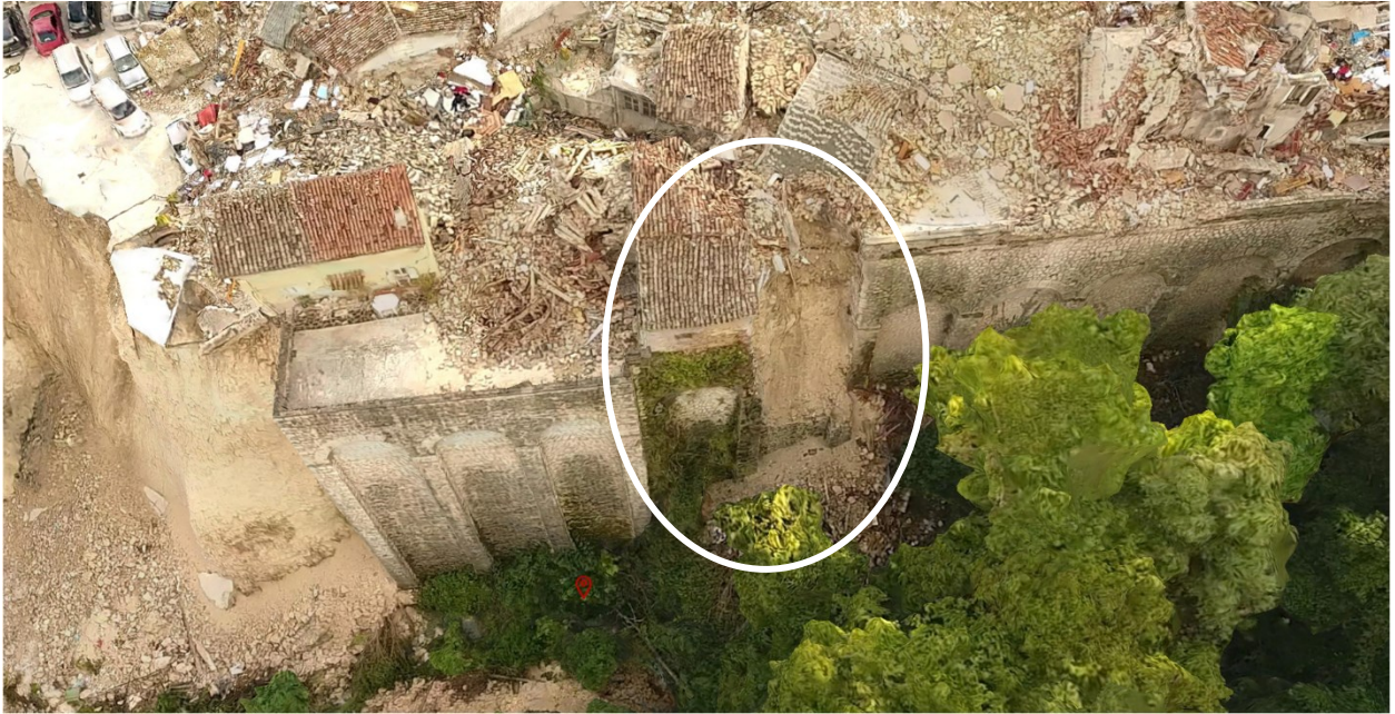
Figure 4.32. Model image of a smaller retaining wall failure and subsequent landslide in Pescara del Tronto (42.75136 N 13.27194 E).
