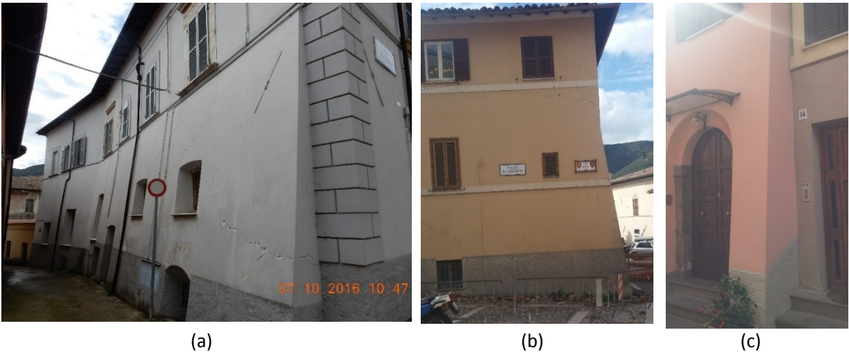
Figure 5.34. Earthquake resistant construction practices in the center of Norcia – linearly varying thickness of the first story.
