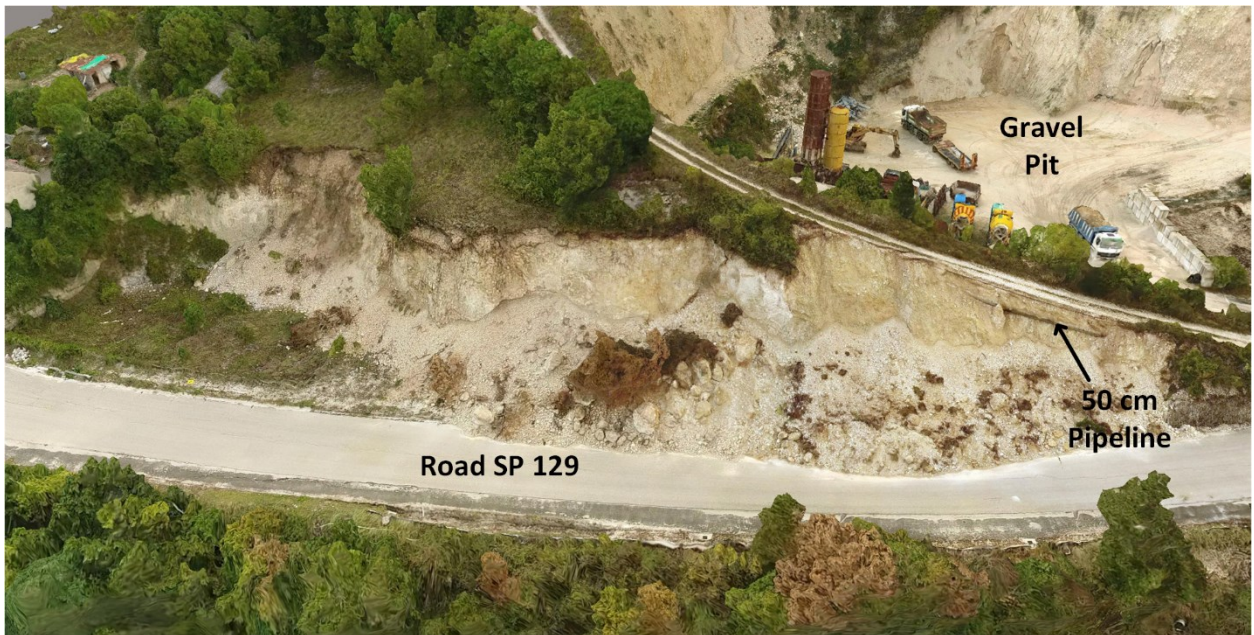
Figure 4.36. Model image of landslide near gravel pit and Road SP 129 that exposed a 50 cm-diameter pipeline (42.74950 N 13.26958 E).
