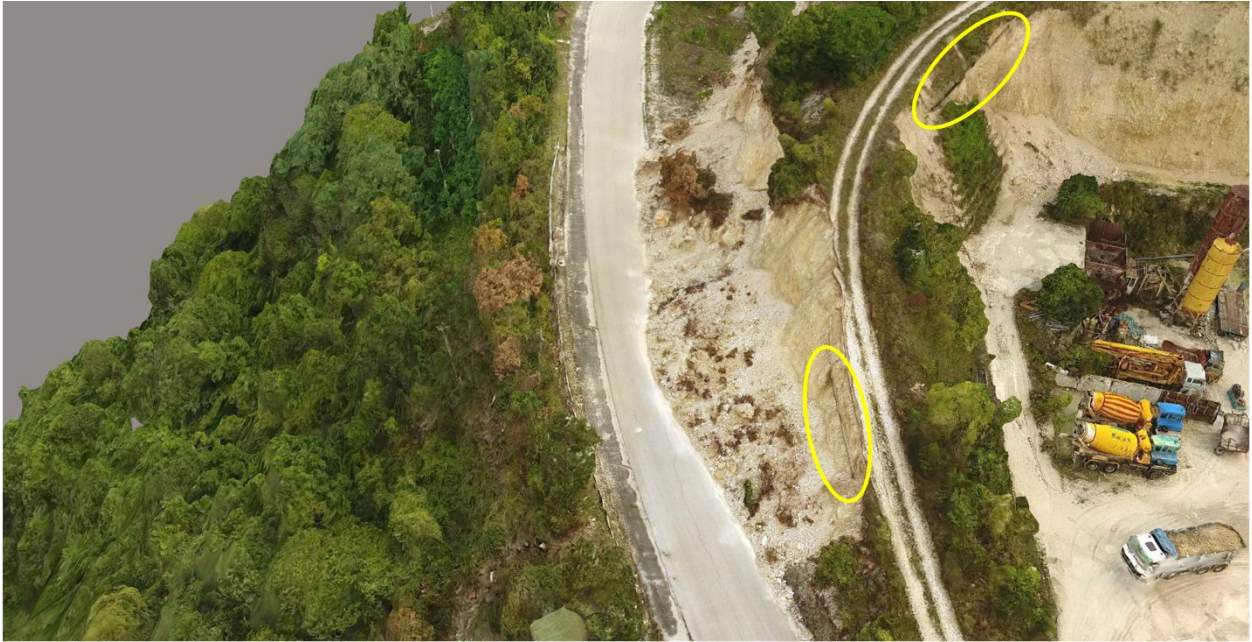
Figure 4.39. Landslides along dirt haul road in Pescara del Tronto, with exposed pipelines. The earthquake caused up portions of the slope up to 5 meters wide to fail, including portions of the dirt haul road itself.
