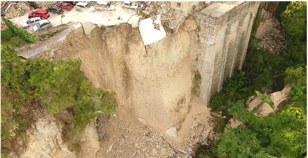
Figure 4.31. Model image of slope failure and possible retaining wall collapse (42.75109 N 13.27208 E).
