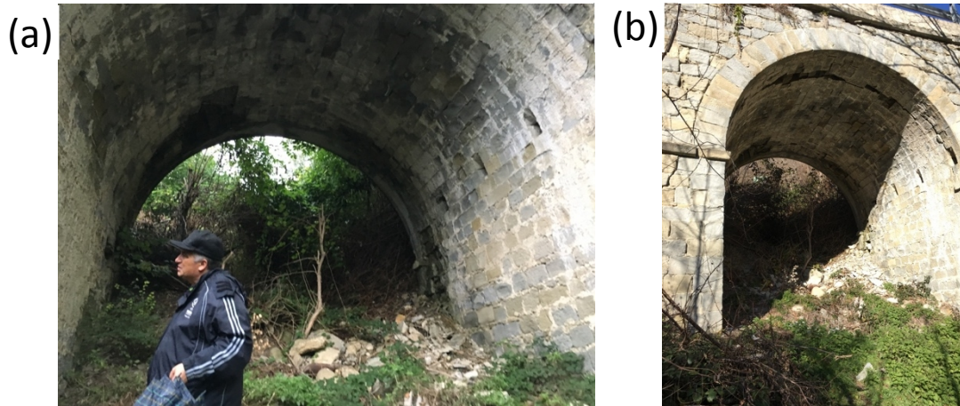
Figure 9. Roman-era bridge along the Trisungo route (1 span bridge - Tufo area – Arquata del Tronto): (a) after the 24 August event (photo on September 7 2016) and (b) after the October events (photo on December 13 2016) (N42.735981, E13.254862).
